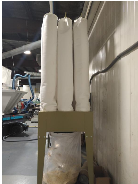
MKOB c/w filter hanger arms & bag waste storage (side)
